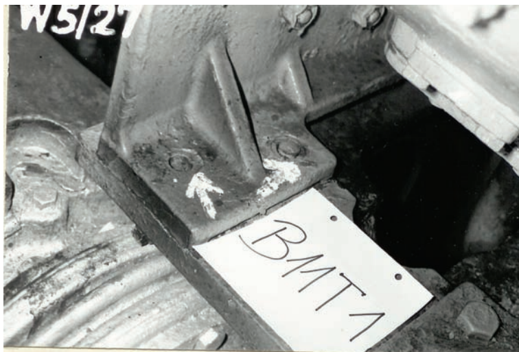
Fig. 2. Foundation bolts torn off the seating of main engine's turbocharger
