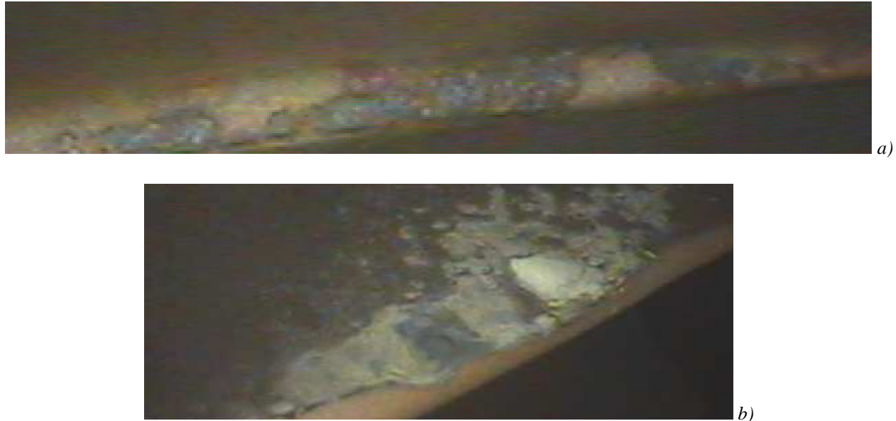
Fig. 3. A part of HP turbine blade of turboprop [7]. a) Sulfur-oxidant corrosion source at LE; b) Corrosion cracks and lack of material made by LE „washing out”
