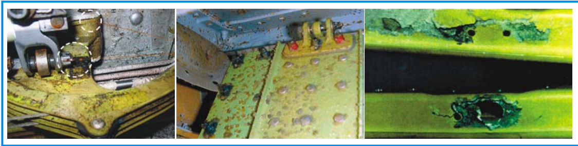
Fig. 5. Types of corrosion – macroscopic image of the surface-layer cross-section
