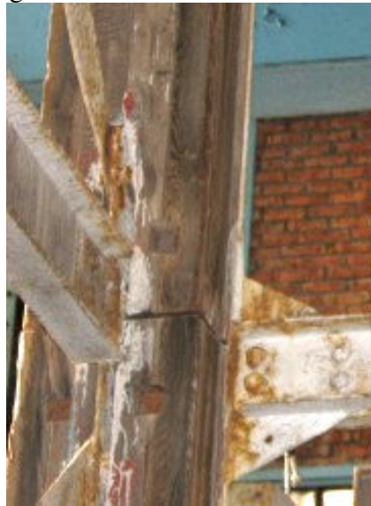
Fig.5. Fragment of the shaft bearing structure with visible traces of corrosion
